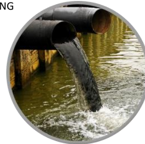
POST WATER TREATMENT
